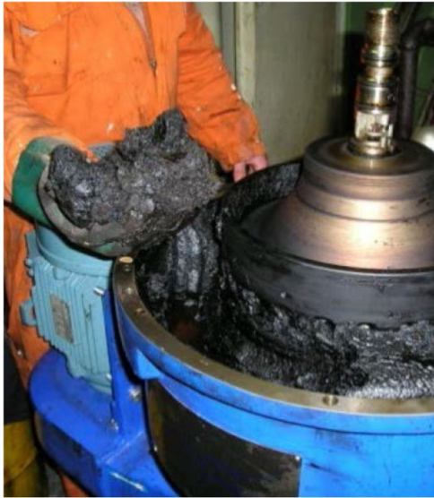
Figure 3: Hybrid Sludge Formation (picture courtesy of DNV-GL)
