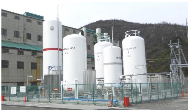
Figure 13: Low-pressure fuel gas supply system (FGSS) for test engine
